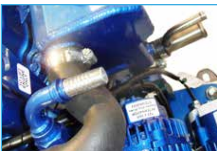
Hot water connections
