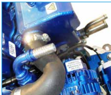
Hot water connections
