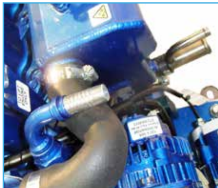
Hot water connections
